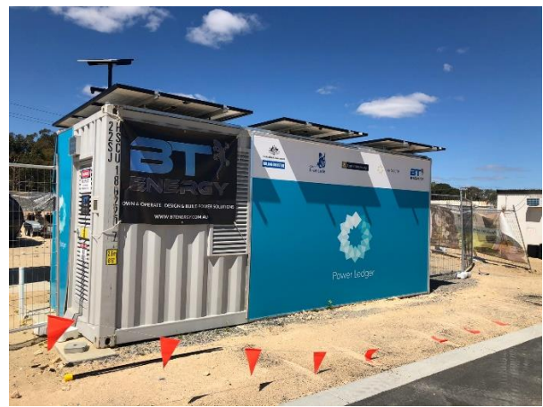
Power Ledger shared battery module installed at site.
