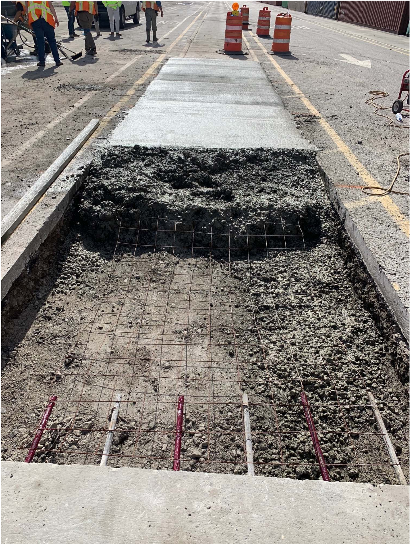
Figure 1. EdenCrete®- enriched concrete being poured at Garden City Terminal, Port of Savannah
