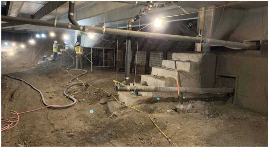
Figure 6. Shotcrete (including EdenCrete®) used in in Health, Nutrition and Physical Therapy Centre
