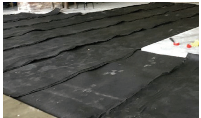
Figure 6. Interior Corridors- 3 inch thick EdenCrete® concrete overlay repair on a drainage system and suspended deck.
