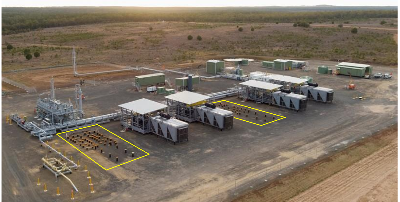
Roma North gas processing facility at 16 TJ/day (~6 PJ/year) nameplate capacity; footings in place (highlighted) ready for expansion to 24 TJ/day (~9 PJ/year)
