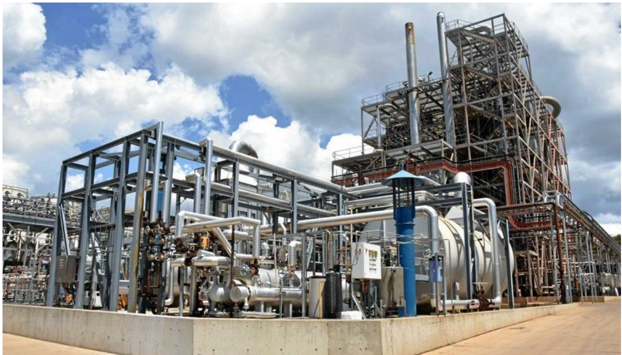
Supplying natural gas to Southern Oil Refining's advanced biofuels and oil refining plants at Yarwun, near Gladstone
