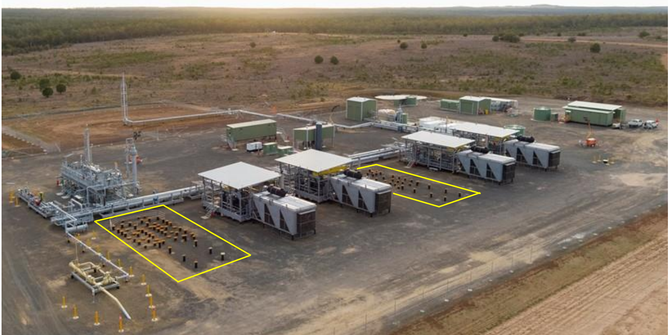
Roma North gas processing facility at 16 TJ/day (~6 PJ/year) nameplate capacity; footings in place (highlighted) ready for expansion to 24 TJ/day (~9 PJ/year)
