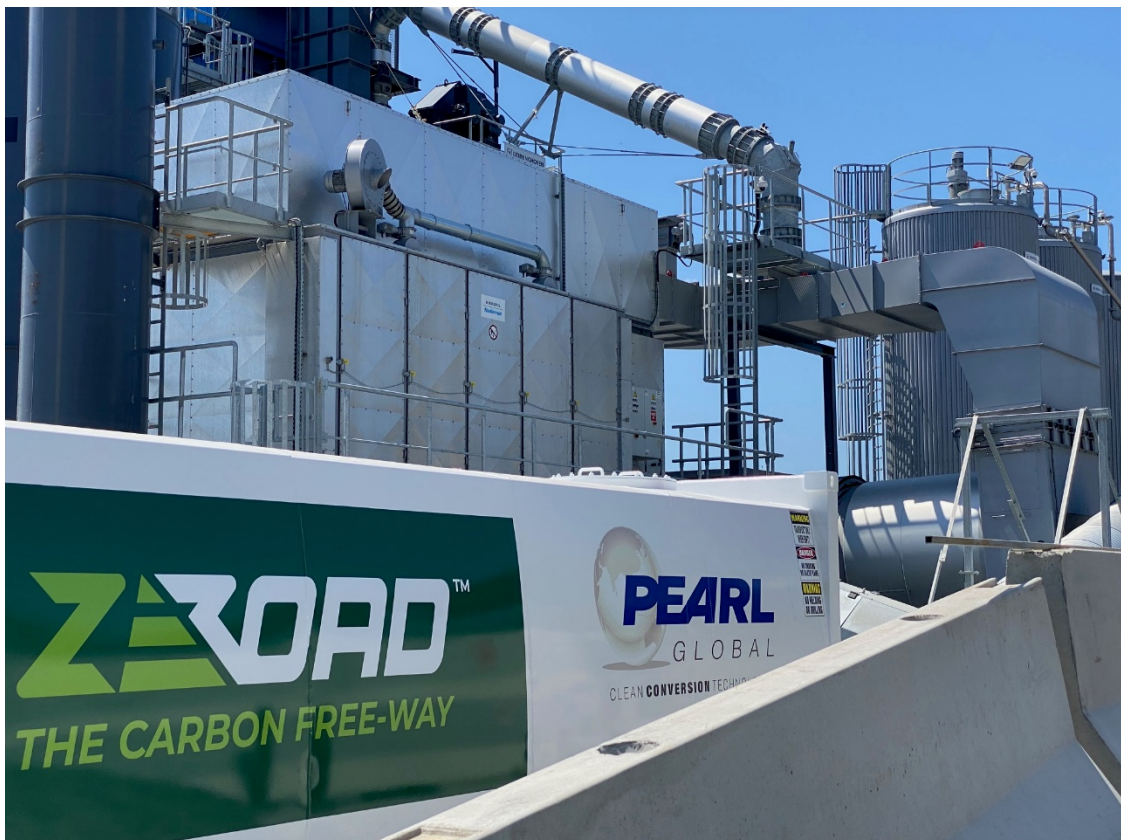
Figure 1: Installation of the tank which will facilitate running of Aussee's asphalt plant exclusively on Pearl Global fuels, showing co-branding of Zeroad and Pearl Global
