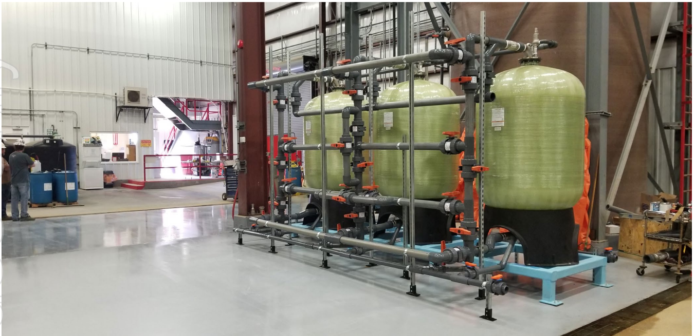
Figure 6: Constructed Ion Exchange Test Columns for MU1A Field Demonstration
