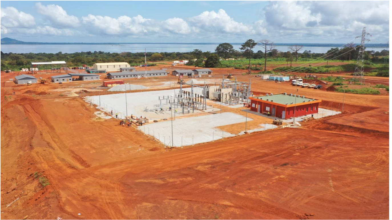
Yaouré substation and switch yard
