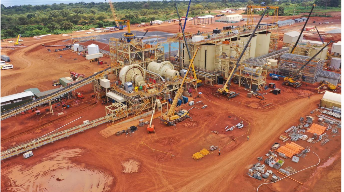
Process Plant including Mill Structure, and CIL tanks
