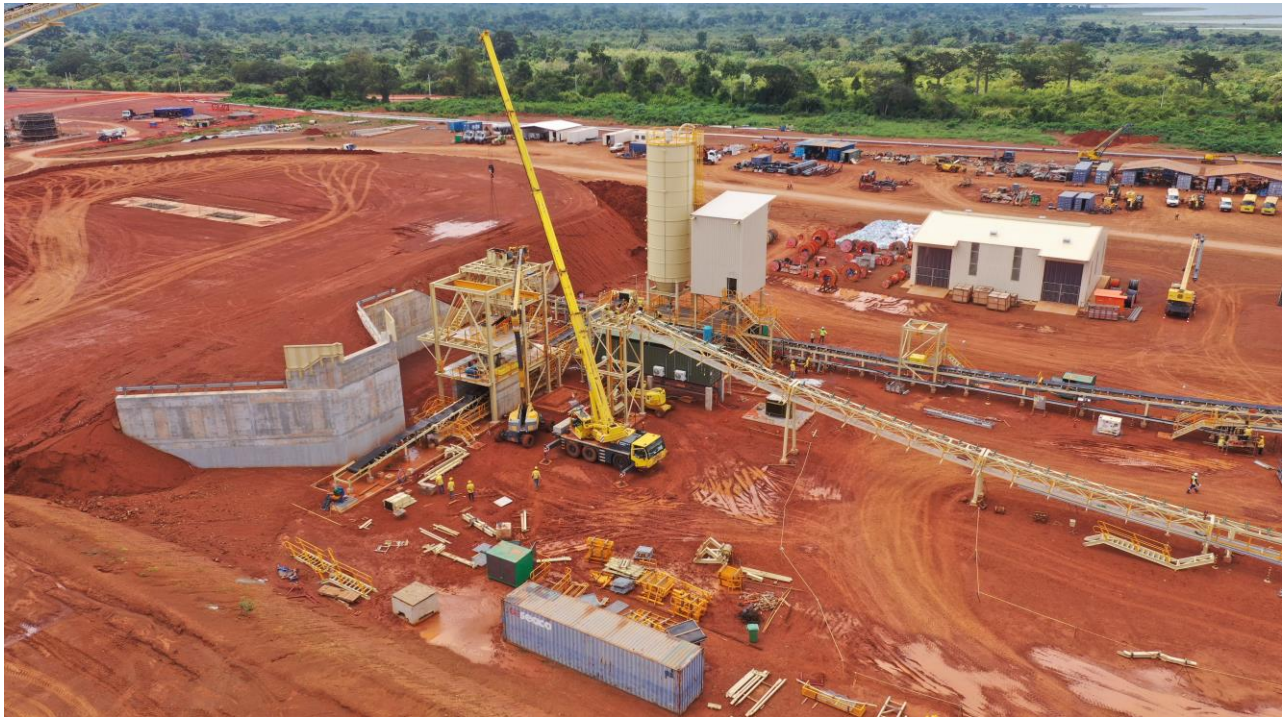
Recycle crushing facility, Lime silo, Reclaim and COS in background
