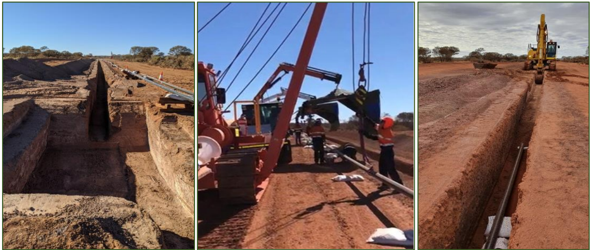
Pipeline trench ready for installation (left), welding of gas pipeline (centre) and pipeline installation (right)
