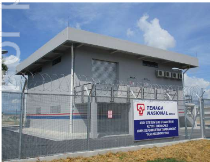
Completed electrical substation, Altech HPA plant site
