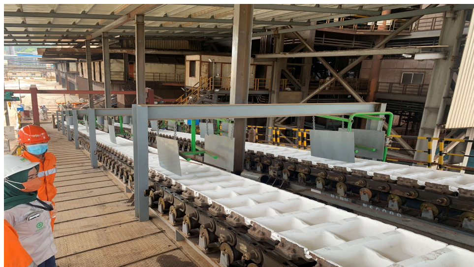
Commissioning of Ingot Conveyer at Ranger Nickel.
