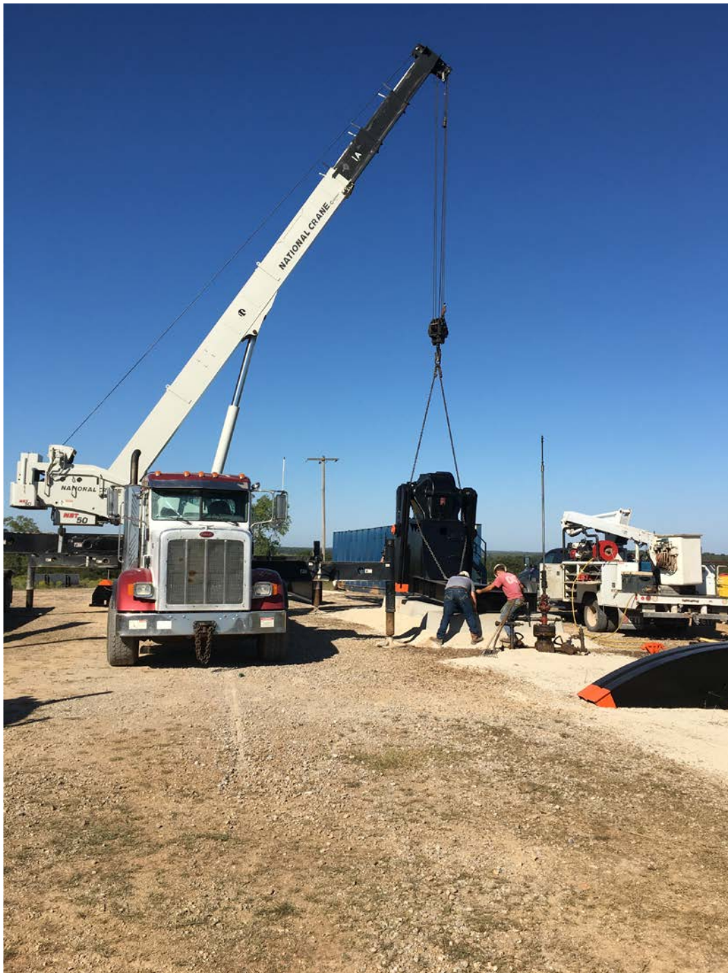
Figure 2. Production equipment being installed on the Mitchell Well in Carter County, Oklahoma
