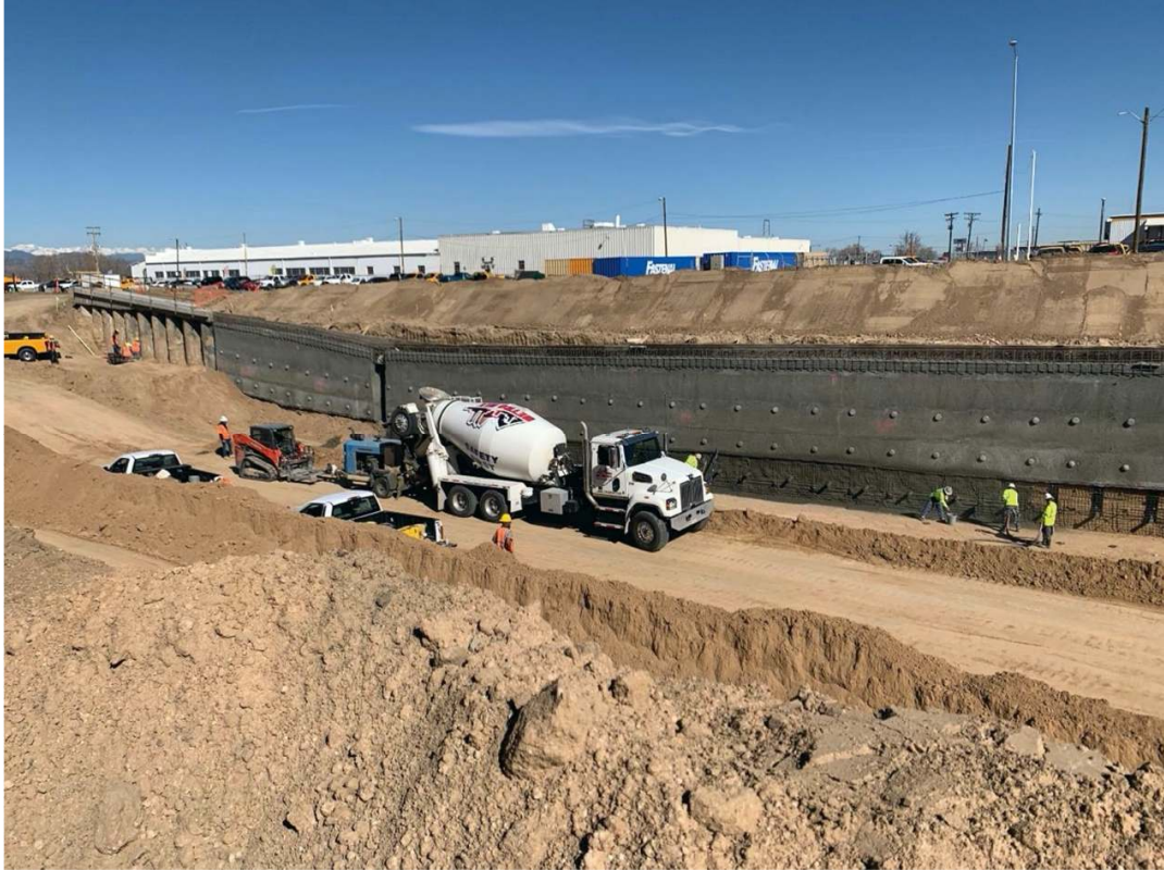
Figure 1. Ground-anchored concrete retaining walls (that incorporate EdenCrete®) along portion of the 10 miles of highway re-construction on Interstate Highway I-70 in Denver.
