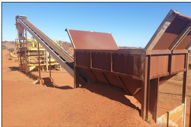
Figure 7. View from feed hopper along feed conveyor to wash-plant.
