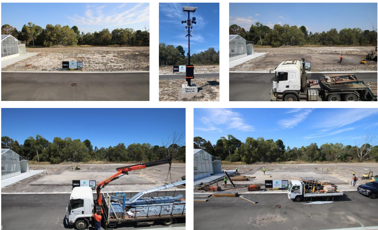
Site preparation and set-out works for the CRC-P partially funded greenhouse commencing at Murdoch University, Western Australia.
