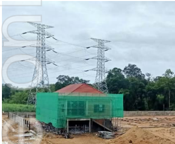
Figure One | Substation Main Control Building
