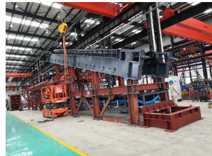
Figure Twenty Two | Apron Feeder for Primary Crusher
