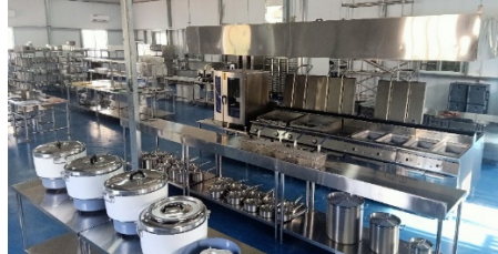
Figure Five | Accommodation Camp Kitchen
