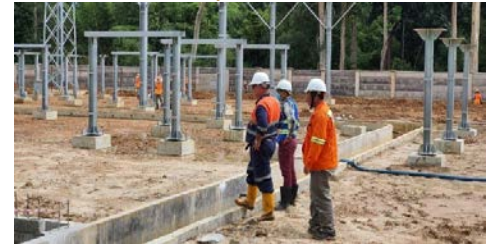
Figure Three | Substation Transformer, Isolator and Bus Bar, Structural Steel Work
