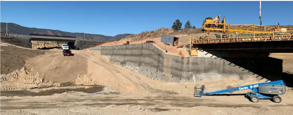
Figure 4. Bridge embutment and retaining wall constructed with EdenCrete® enriched concrete
