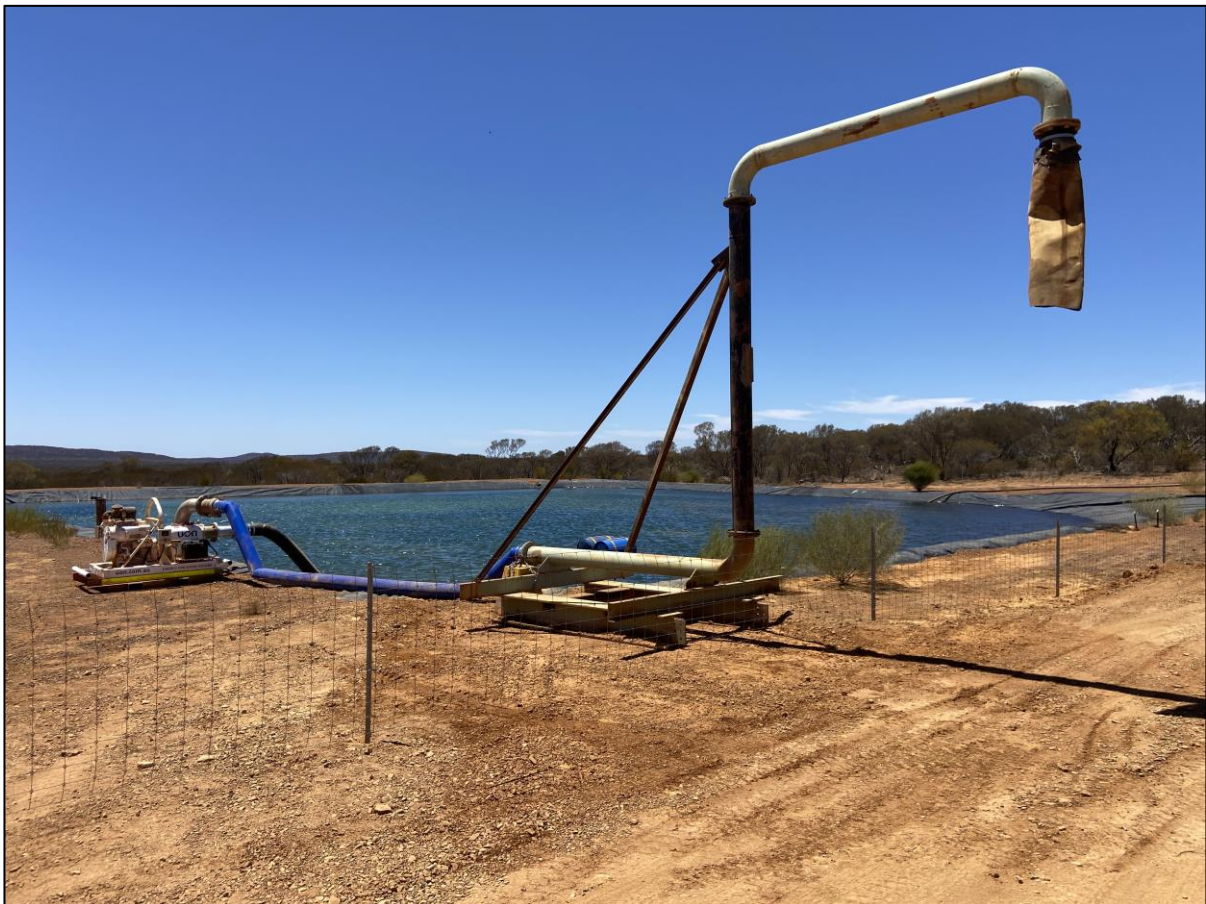
Figure 2: Site water supply established at the Shine Iron Ore Project as part of early siteworks.
