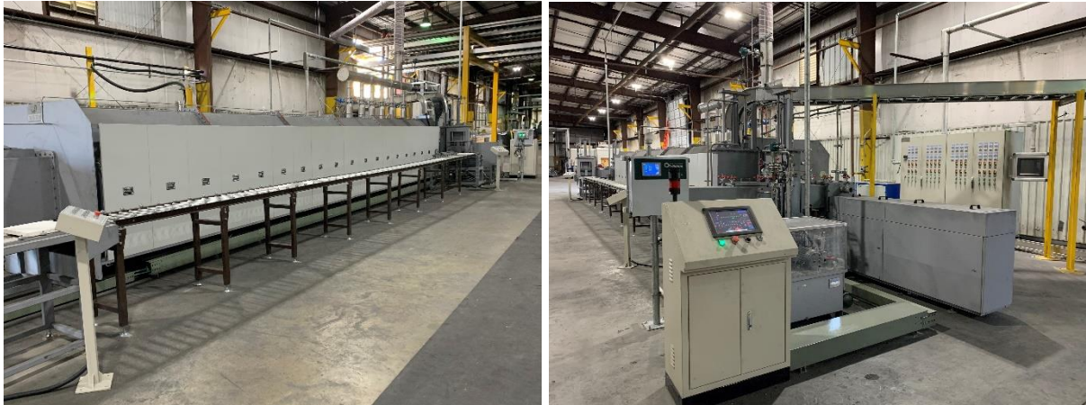
Figure 1: Main furnace chamber (left) and furnace control station (right) at Vidalia.
