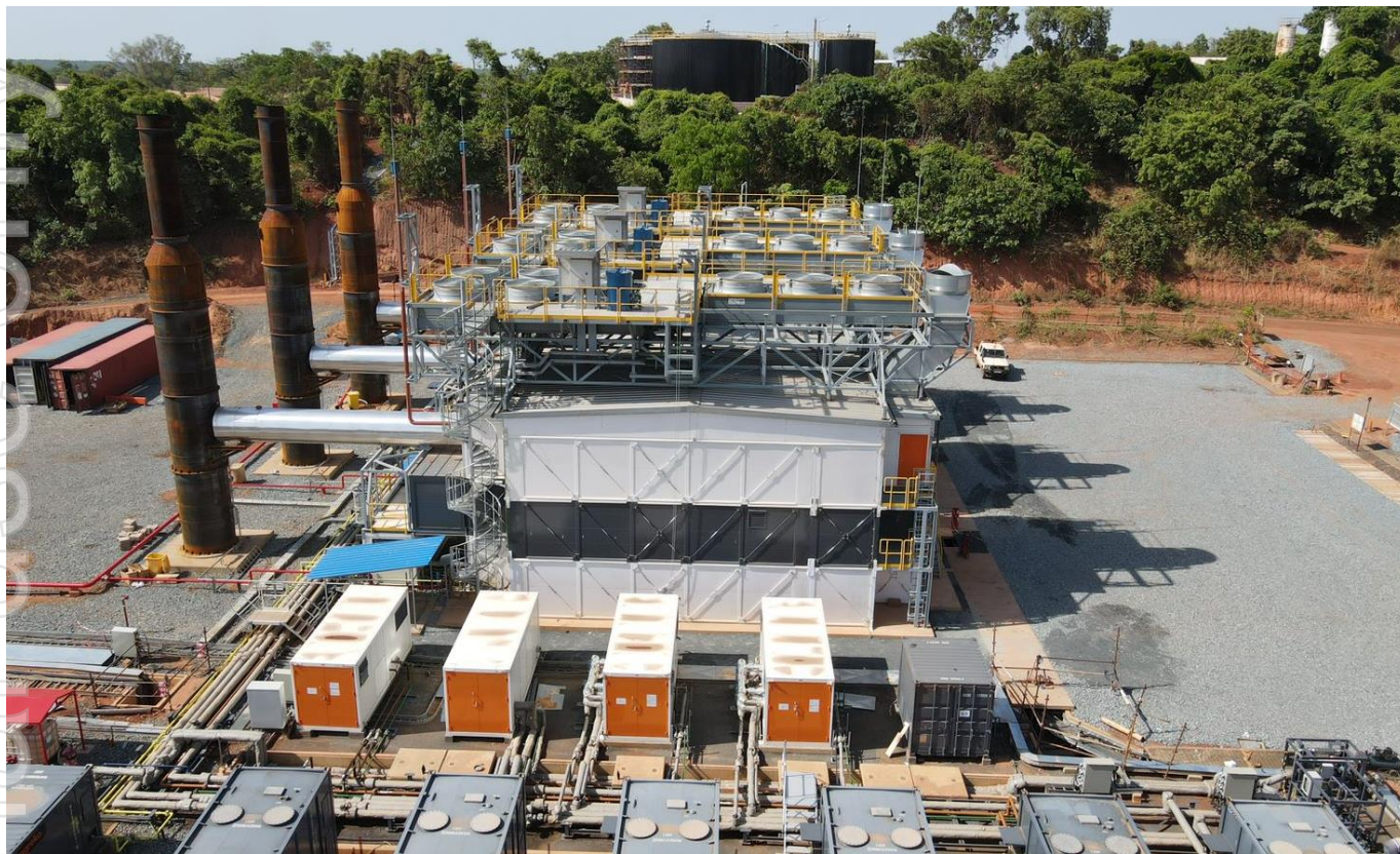
Figure 1: Completed Syama Hybrid Power Station with HFO storage in background
