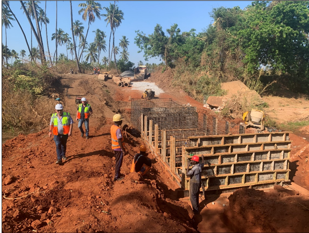
Figure 3: Allan Mulligan (COO) and Bruce White (PM) inspecting the construction by TNR of the Tanroads designed Low Water Bridge over the stream near Ruangwa.
