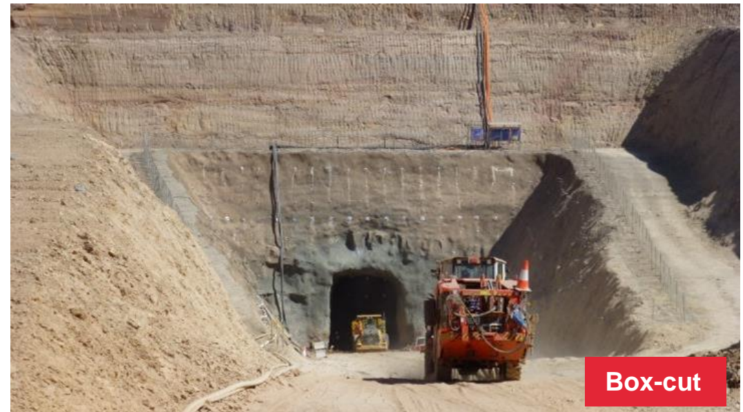
280-unit mine site village
