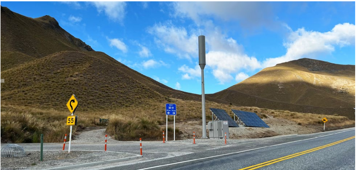
RCG cell tower at Lindis Pass providing mobile coverage for 4km of State Highway 73, powered by 36 solar panels.
