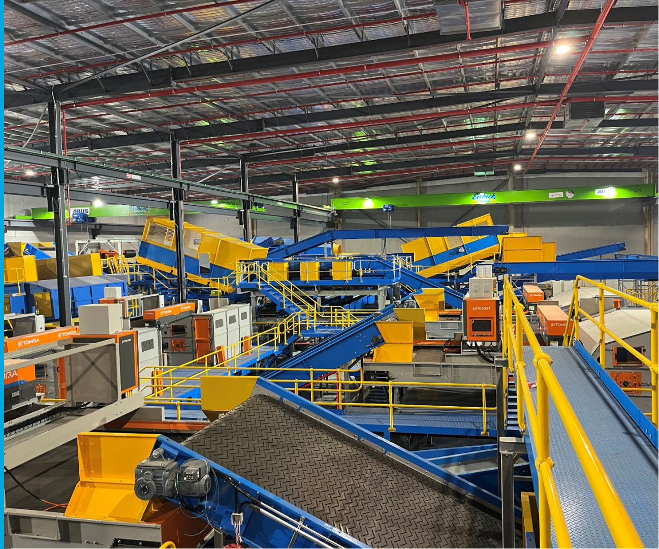
Pictured: Inside Western Sydney MRF pre-commissioning
