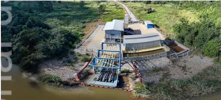
Water collection system in Valadares
