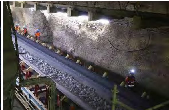
First ore on Conveyor to Surface belt in October 2024
