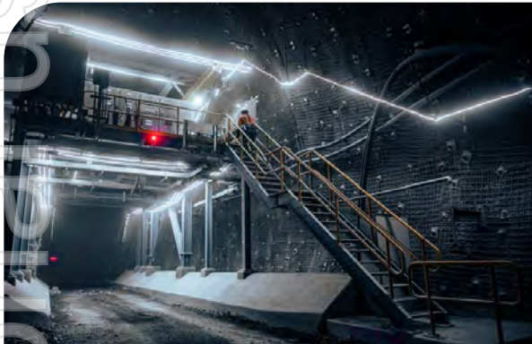
Panel 0 Material Handling System complete
