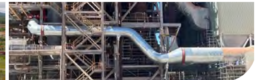
Hydrogen calcination pilot Construction is underway at Yarwun for this world first technology
