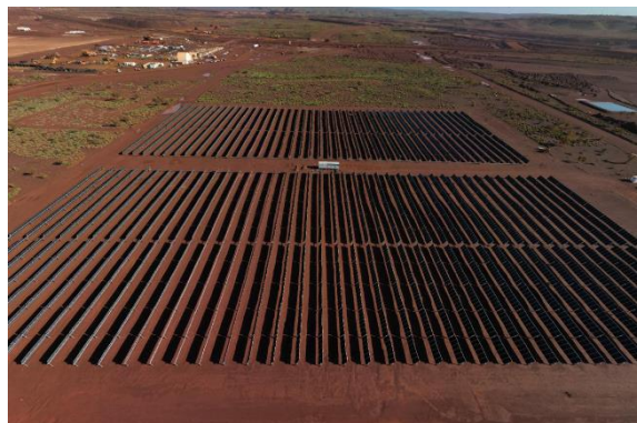
Solar array at Ken's Bore
