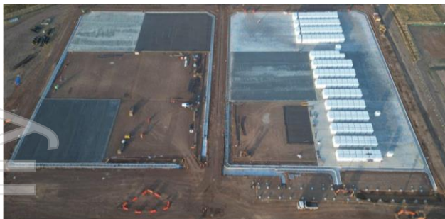
Picture: Mortlake battery
