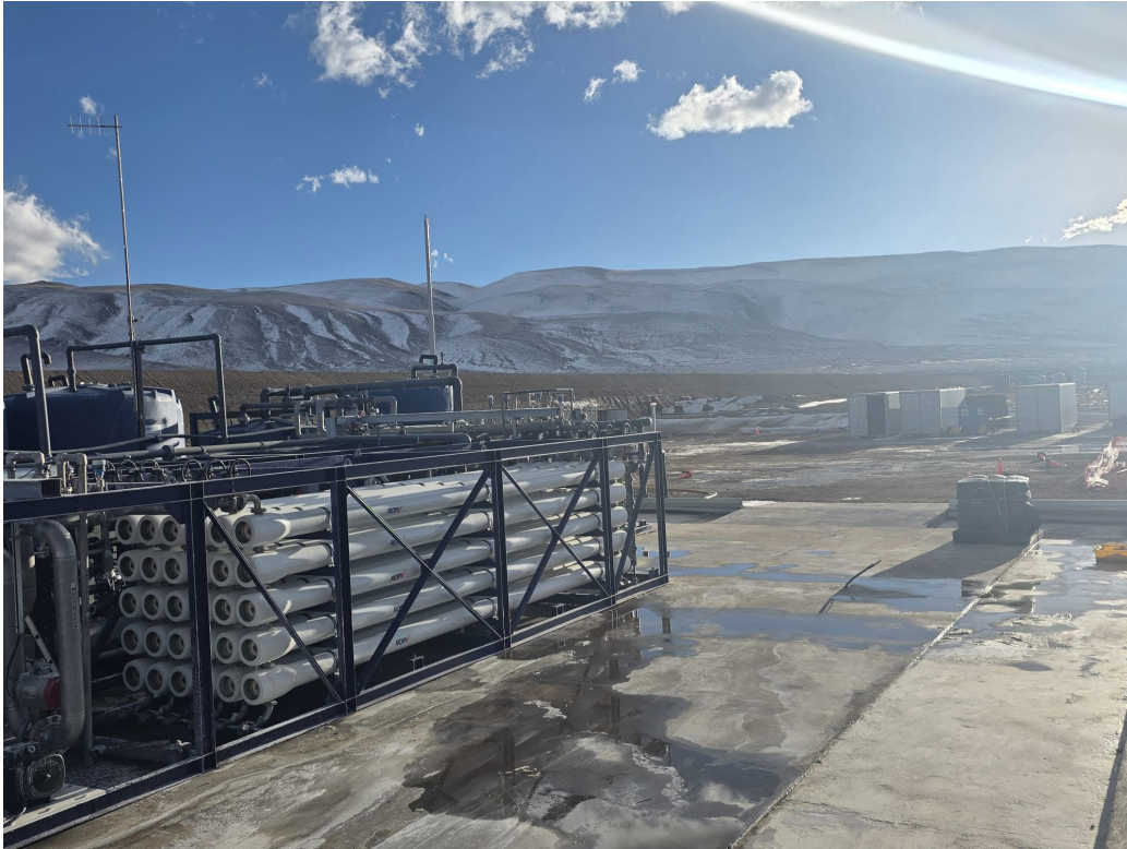
Figure 2. Operational HMW nanofiltration plant.
