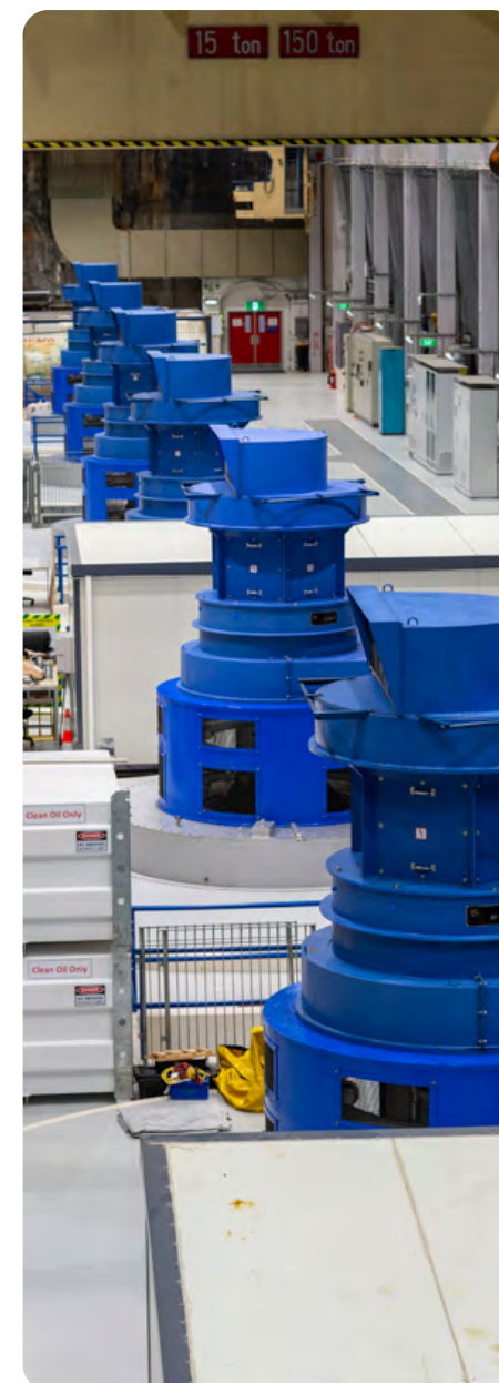
ABOVE: Manapōuri Power Station, Fiordland.
