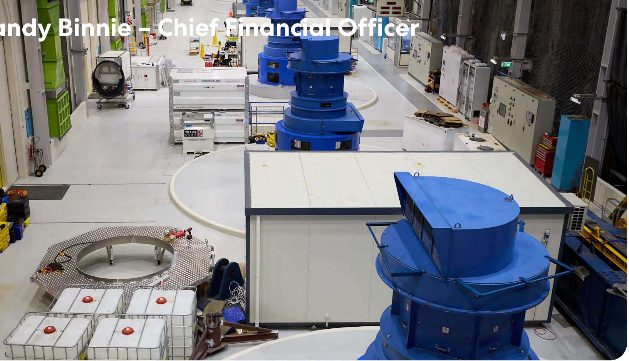
Meridian's Manapouri hydro power station
