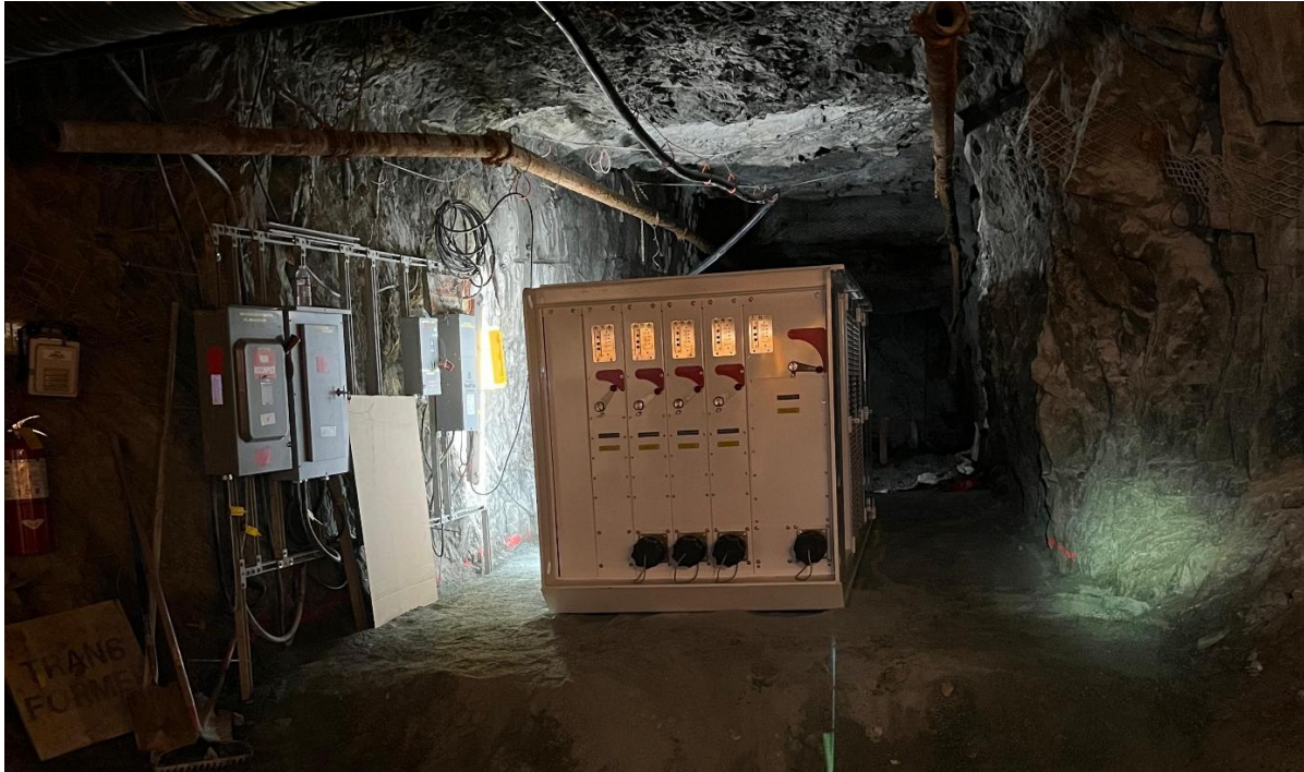
Figure 2: New underground Mine Power Centre installed at XC7, 3 September 2026.
