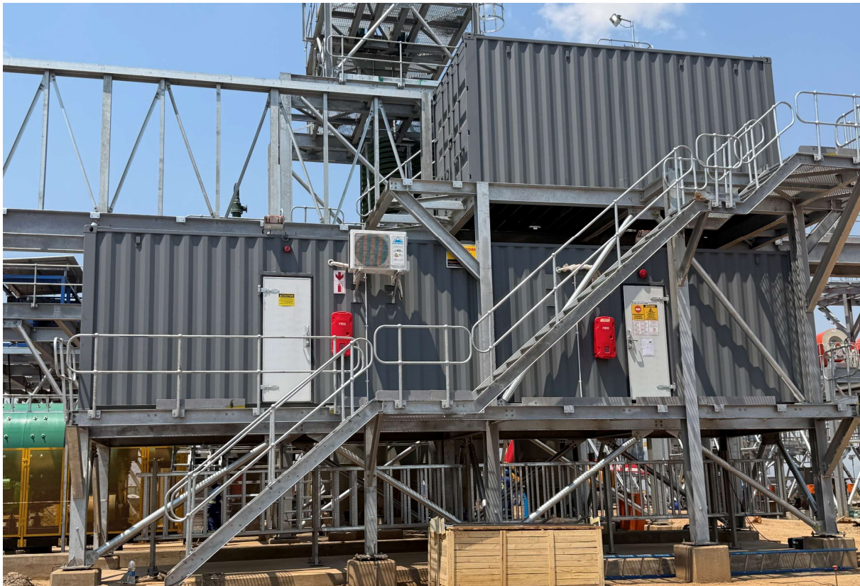
Picture 3. Installed motor control centres at the Kangankunde process plant ahead of electrical commissioning
