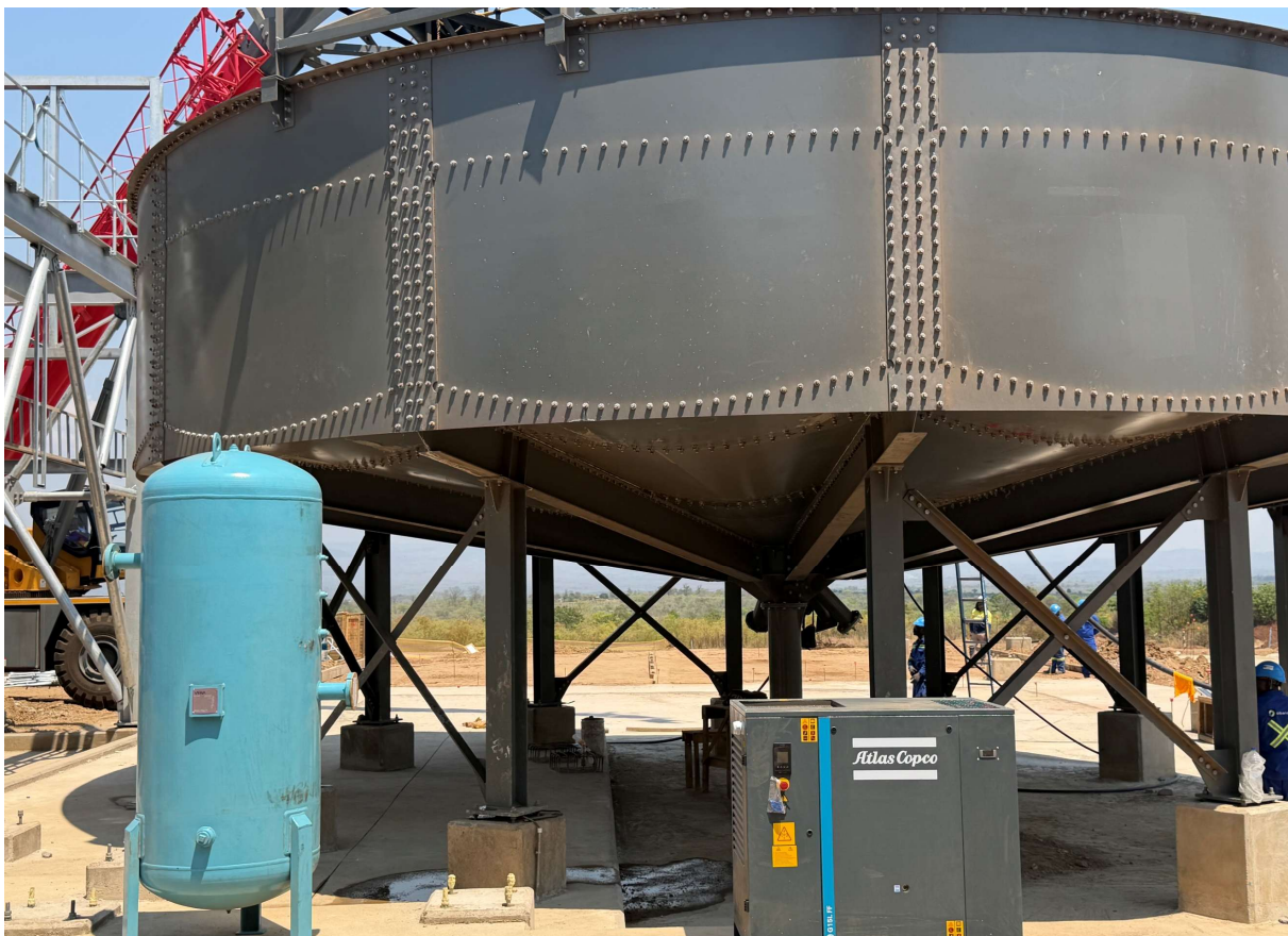
Picture 9. Thickener installed at the Kangankunde process plant ahead of staged commissioning
