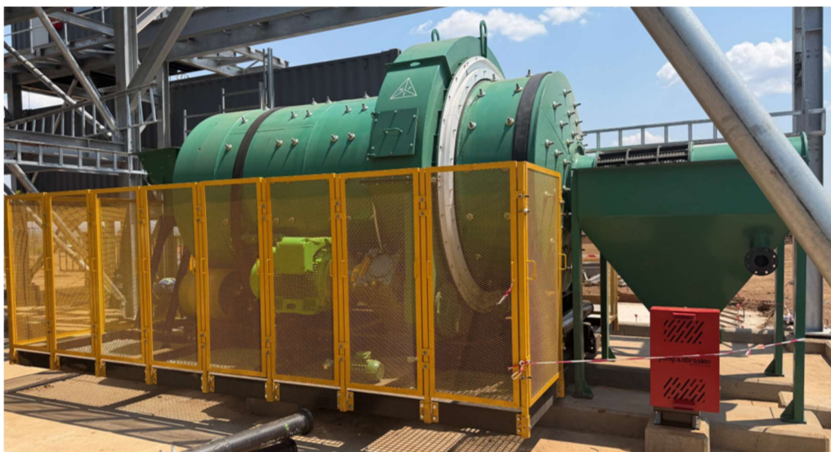
Picture 2. Regrind Mill installed at the process plant at Kangankunde
